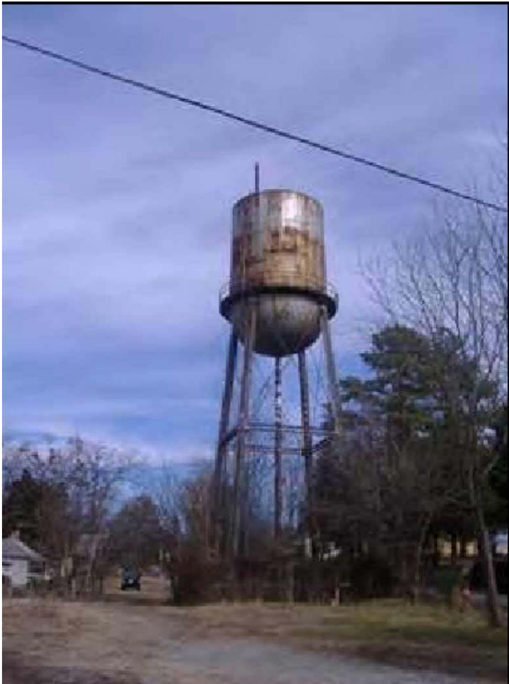
The water tank (fire protection only)
